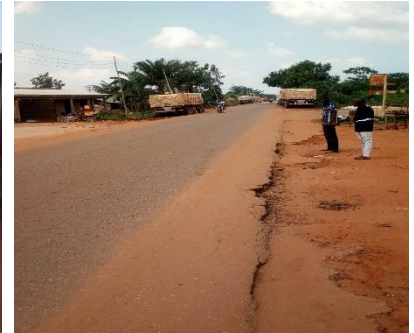
Plate 6: Road without drainage in Ohunbe
